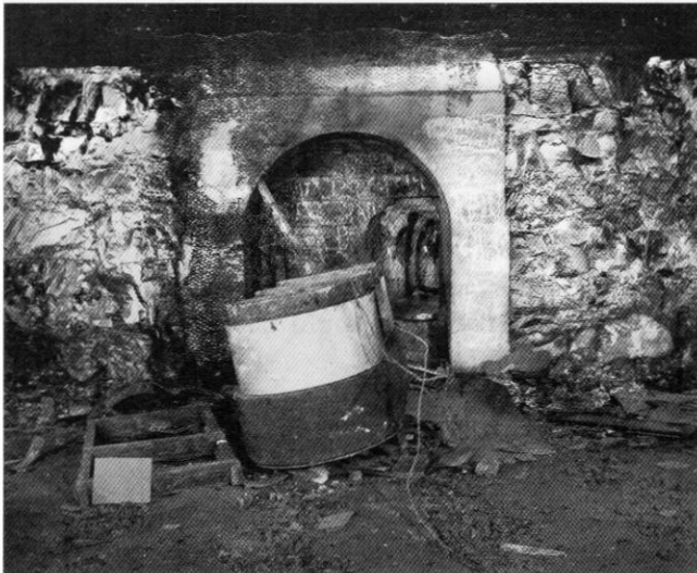
Entrance to the new shelter tunnels from the standard-gauge railway tunnel which was also part of the shelter
